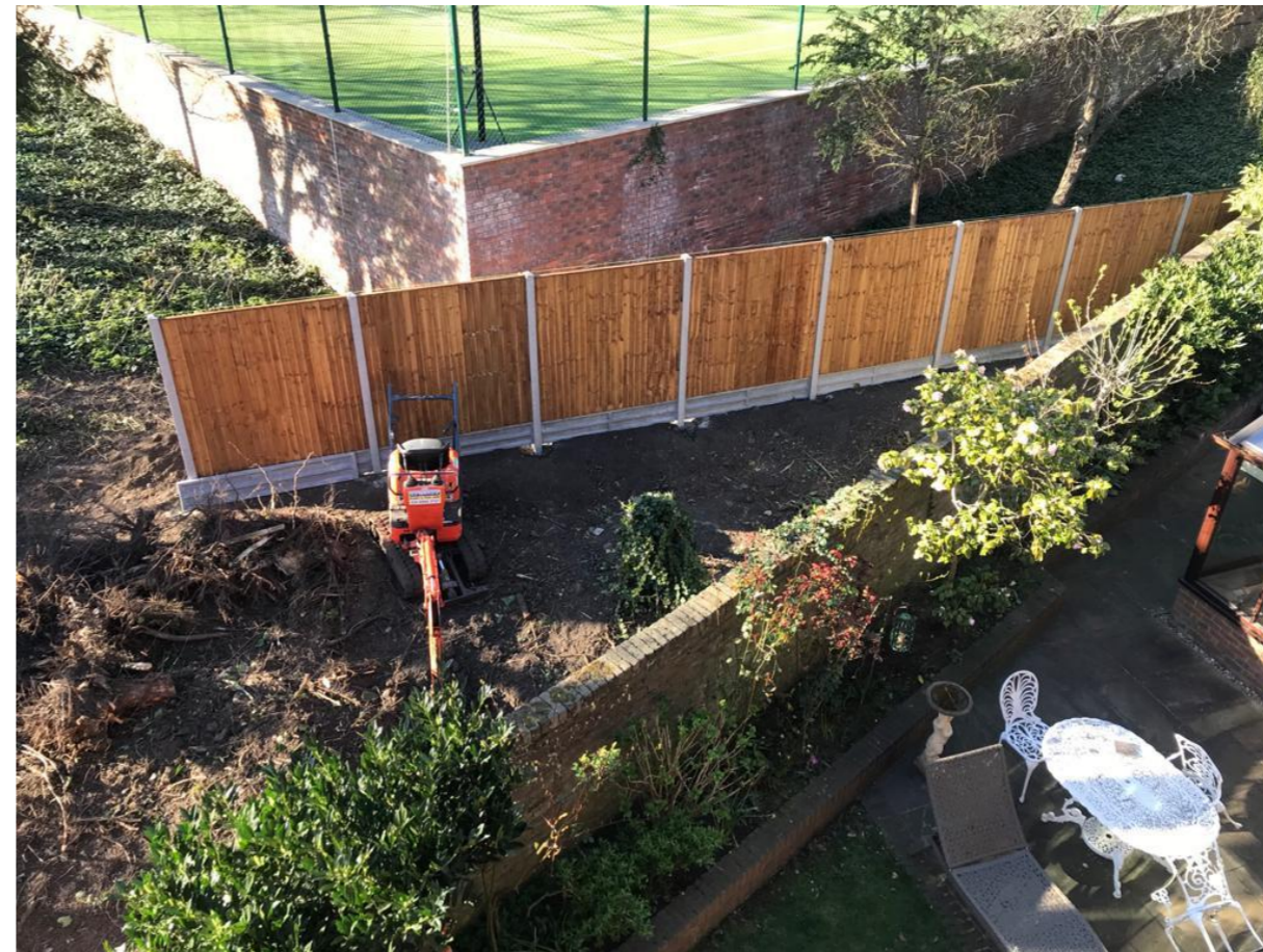
Figure 2 Photograph of the former brick boundary wall and partial completion of the new timber boundary fence
