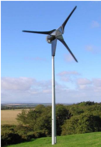
Figure 11 Typical wind turbine.
