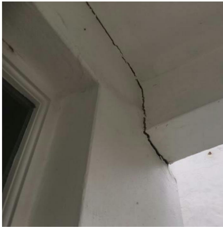
Cracking to porch
