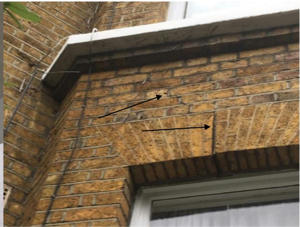
Cracking to bay
