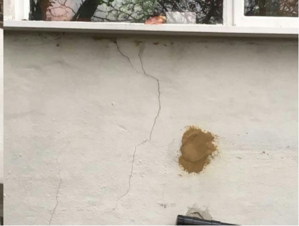
Cracking to rear elevation
