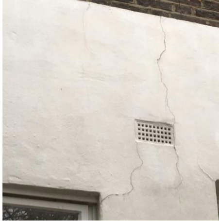
Cracking to rear elevation
