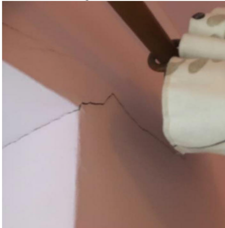
Rear Bedroom - Garden floor flat - rear wall
