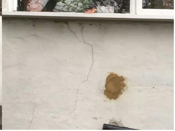
Cracking to rear elevation
