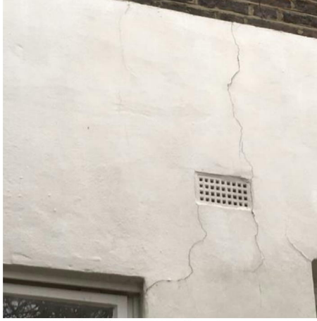
Cracking to rear elevation
