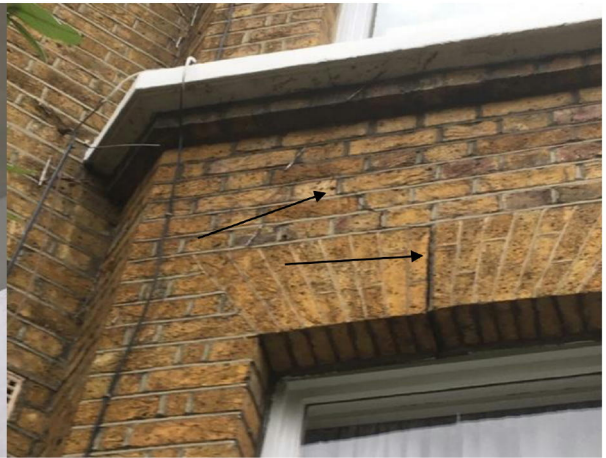
Cracking to bay
