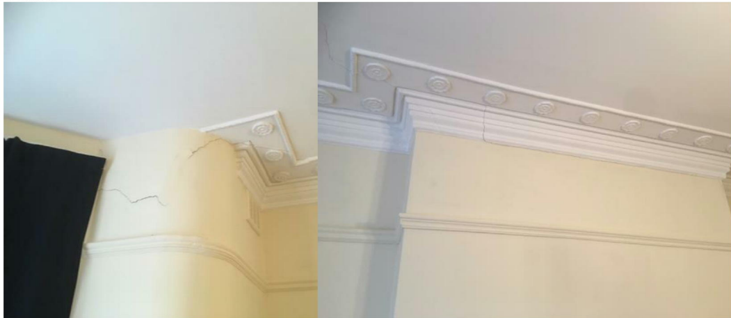
Cracking to first floor flat
