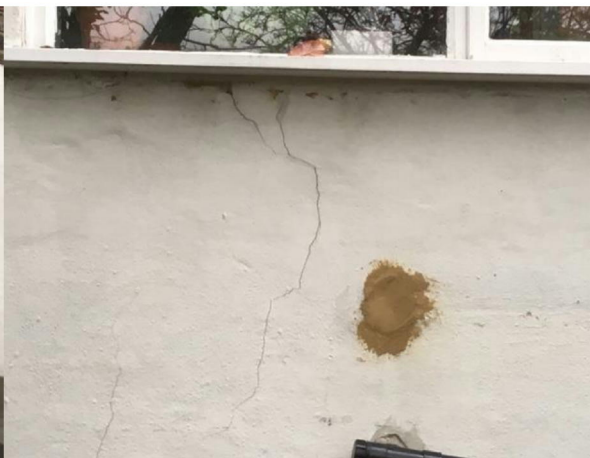
Cracking to rear elevation
