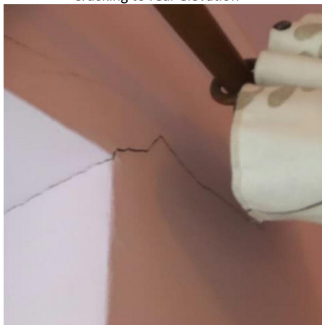
Rear Bedroom - Garden floor flat - rear wall
