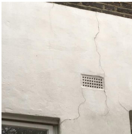
Cracking to rear elevation
