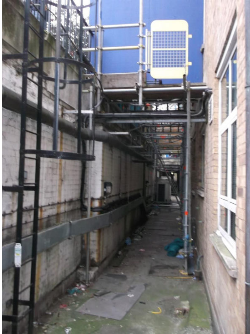
Plate 8: View of a light well showing the street level of Great Ormond Street and the basement level of the Frontage Building, looking south-west
