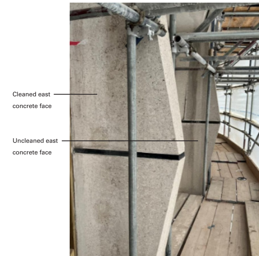
Fig. 2.1.5 East concrete faces (cleaned and uncleaned)
