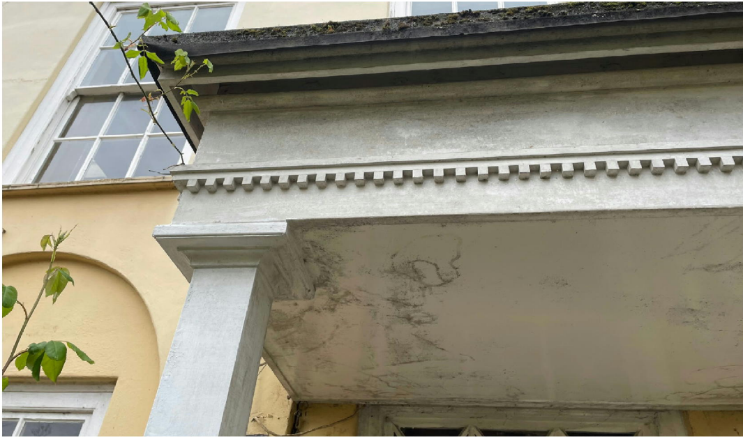
Poor quality timber canopy with asphalt roofing over
