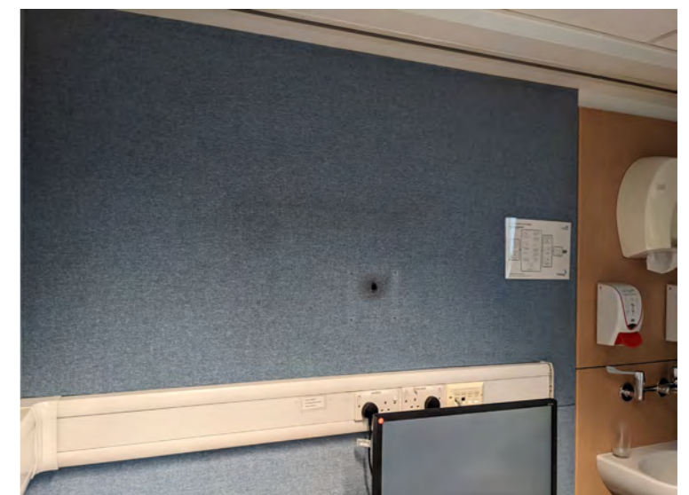
ad hoc electrical services - replacement of fuse boards required to comply with British Standards
