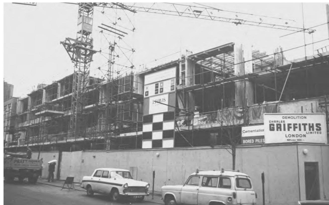
Second phase Frontage building construction, 1968 (note alternative vertical structural strategy with fin walls creating hollows for services)
