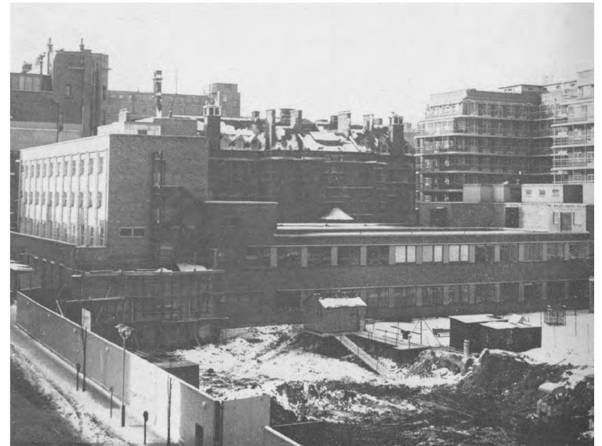
The demolition of the remaining Georgian terrace to make way for the second phase of the Frontage Building 1968
