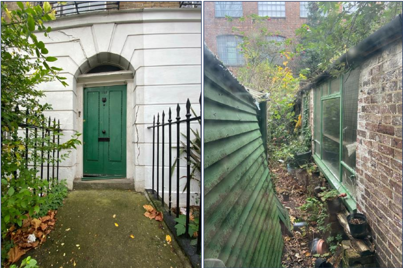
Figure 3- Photograph showing the condition of the existing front entrance (left) and rear outrigger and outbuilding (right)
