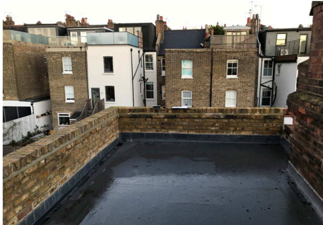
View of existing flat roof: looking towards the rear of houses in Gladys Road.
