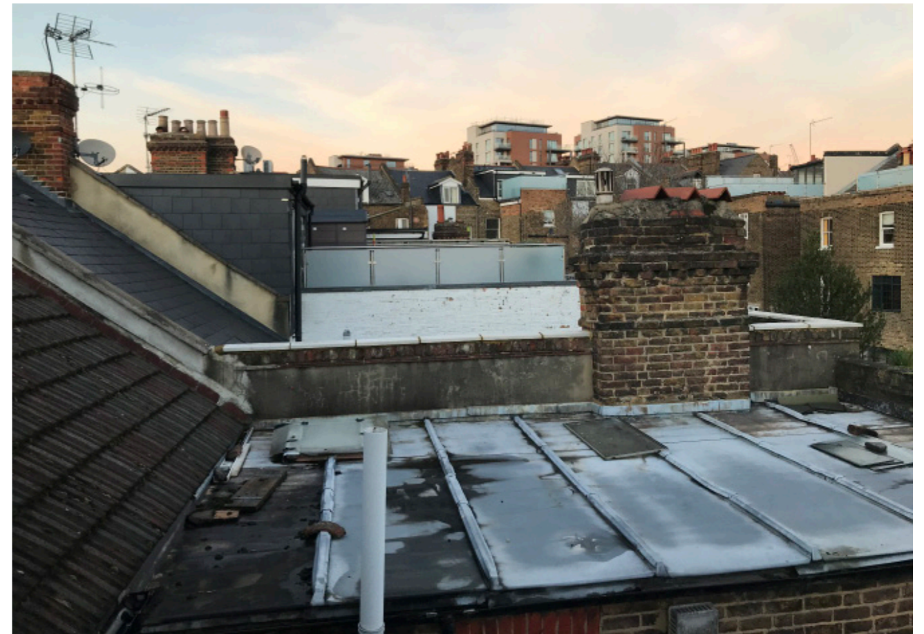
View from roof of 13 Kylemore Road towards roof terrace at no.7 Kylemore Road.
