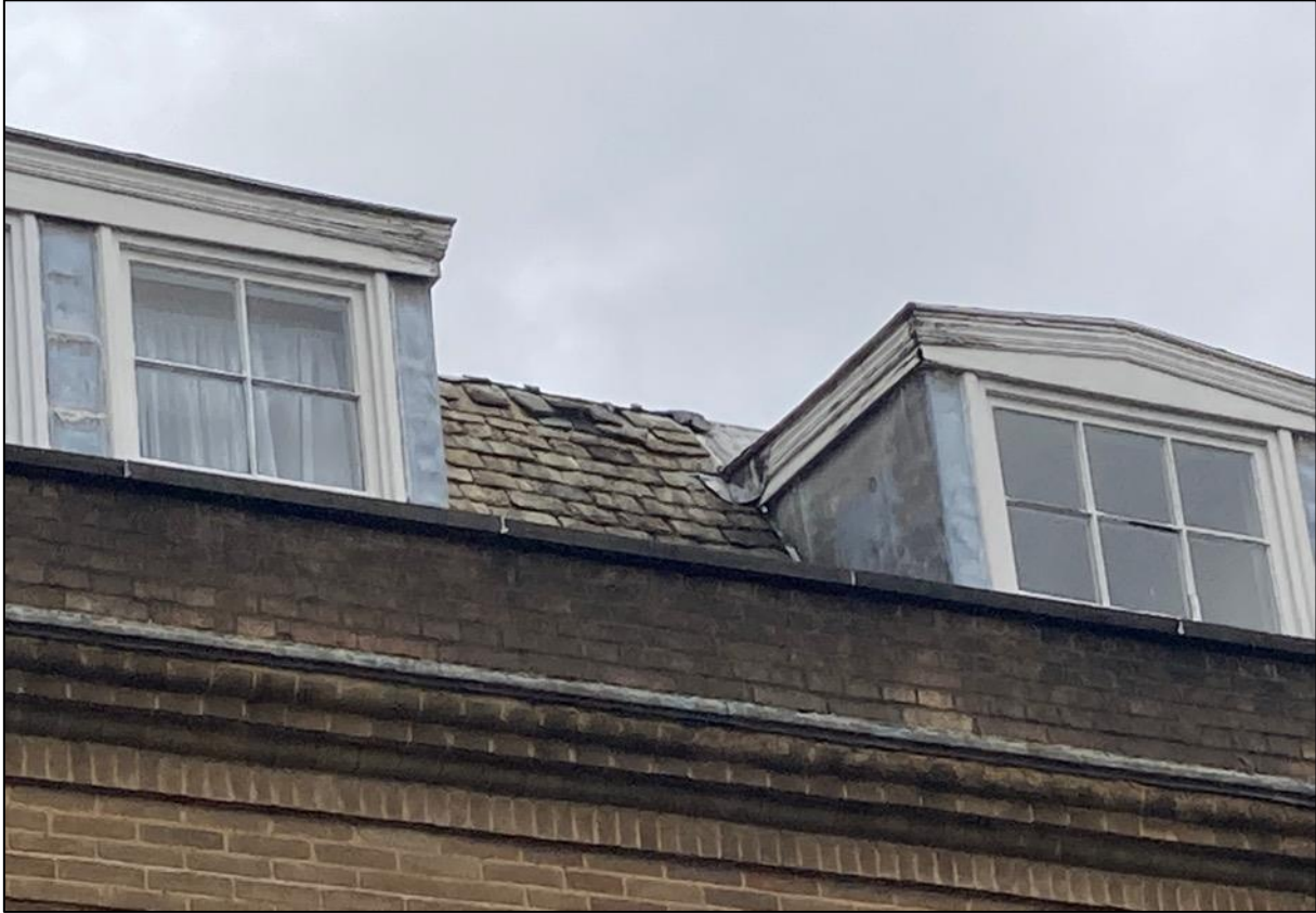
Photograph 2. An area of loose slate tiles at the south-western aspect of the dwelling's roof.
