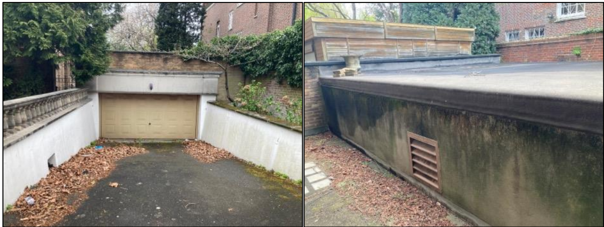
Photograph 5a (left) & 5b (right). Left – the garage viewed from the south-west. Right – roof of the garage viewed from the north-west.
