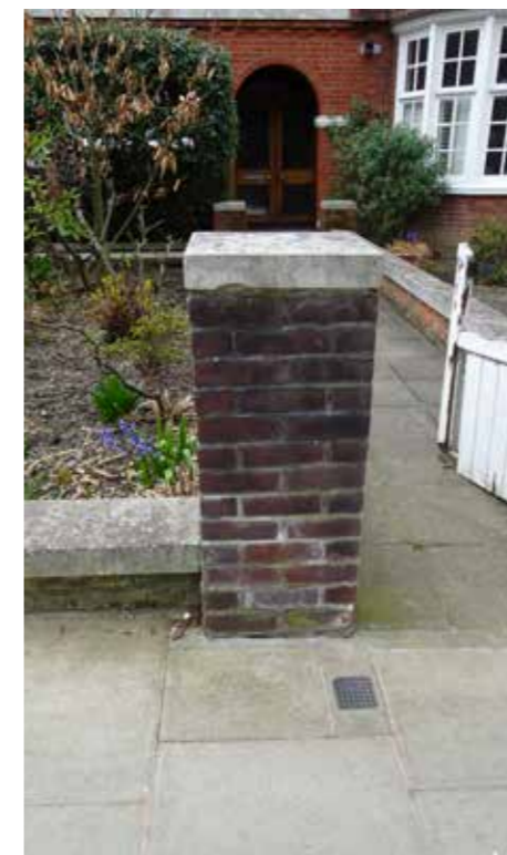
Above: Entrance gate needs to be replaced and pillars re-pointed for consistency,
