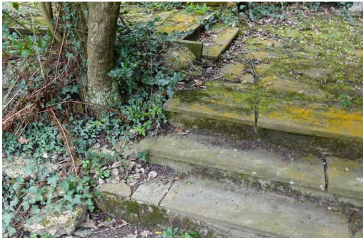
Above: Broken paving and existing poor planting/hazards. As part of the proposals, the long walk will be fully refurbished and replanted.
