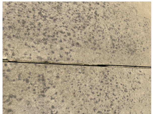
Figure 4: open joints in Bathstone steps
