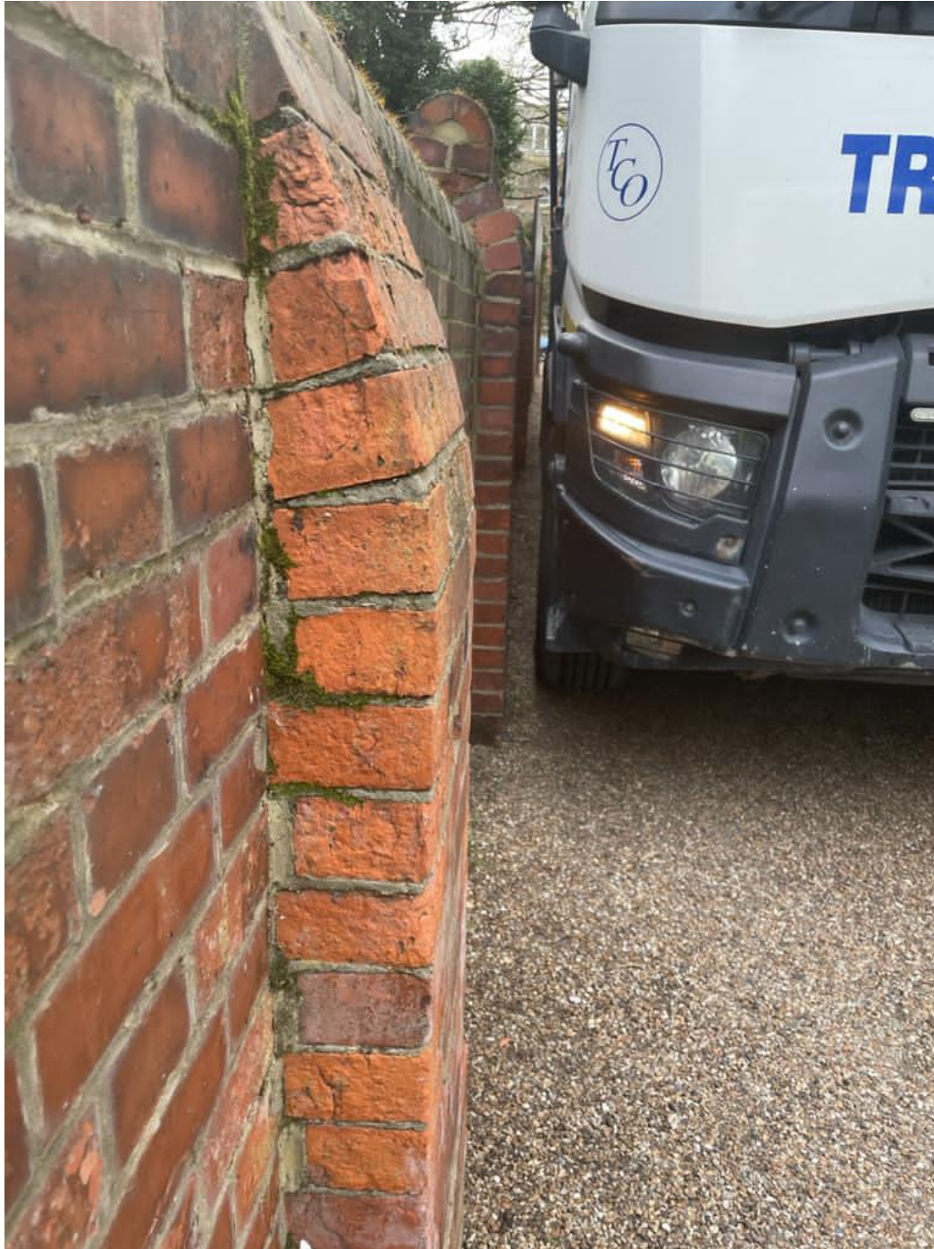
Proximity of a construction vehicle to the Spring Walk boundary wall
