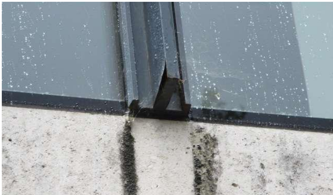
6. Photo showing corrosion and uplifting finishes to the First Floor Oriel Bay Windows.
