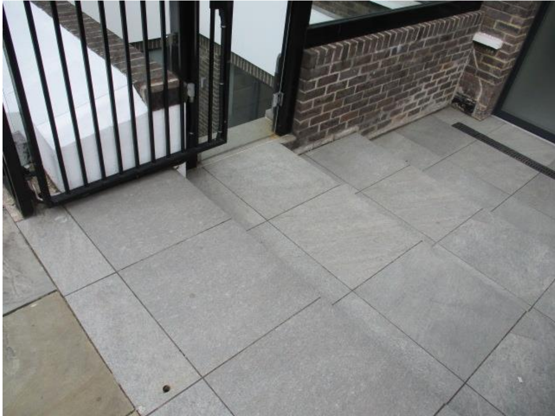
7. Photo showing the obstructed fire escape from the basement lightwell.
