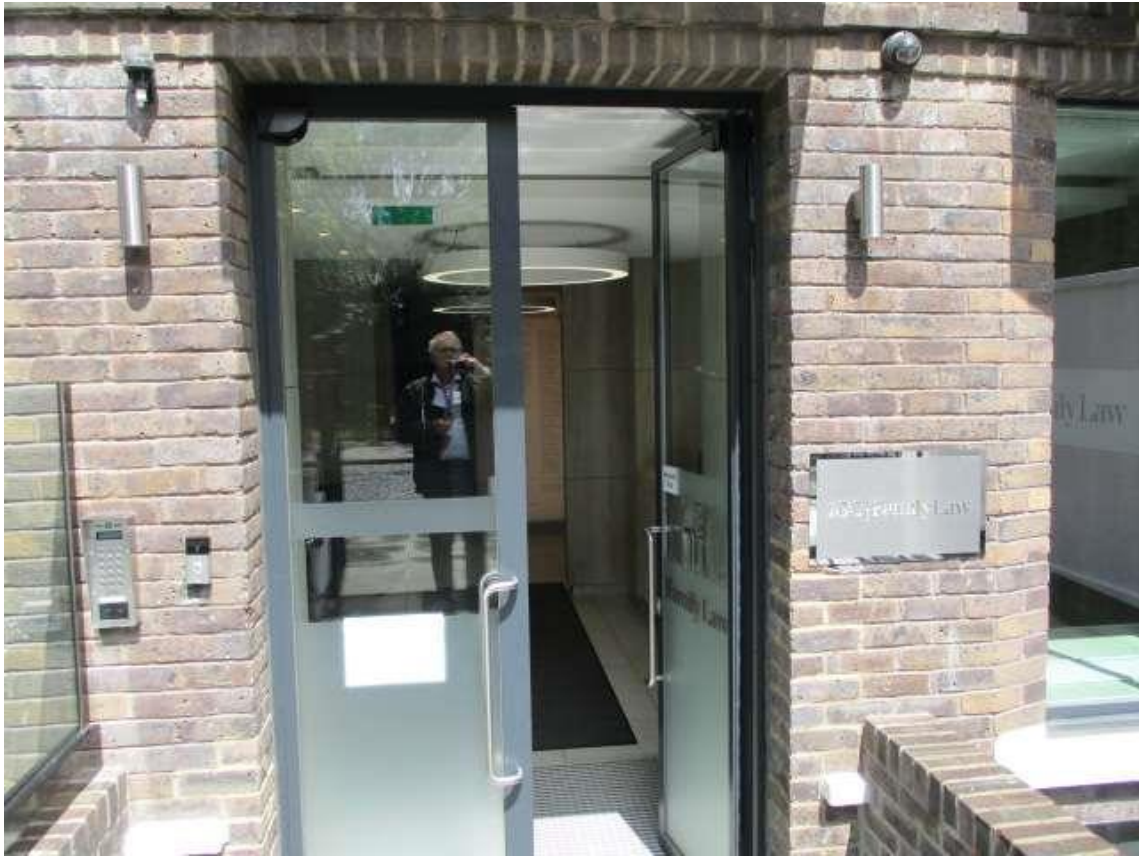
5. Photo showing Front entrance doors not complying with means of escape regulations.
