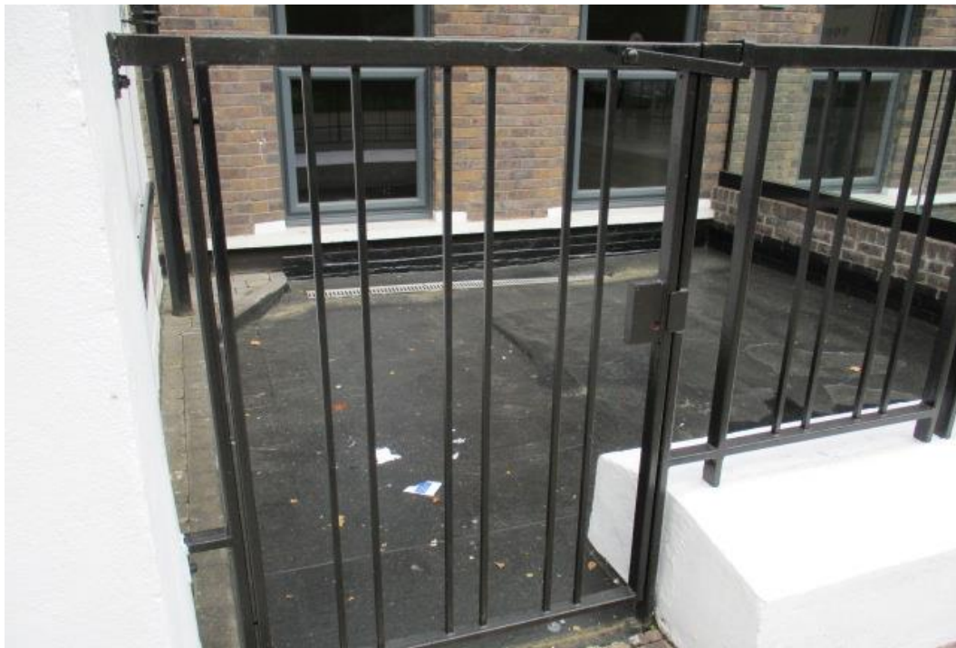
8. Photo showing the current opening to Roof A. This is to be adjusted to comply with the S106 Agreement.
