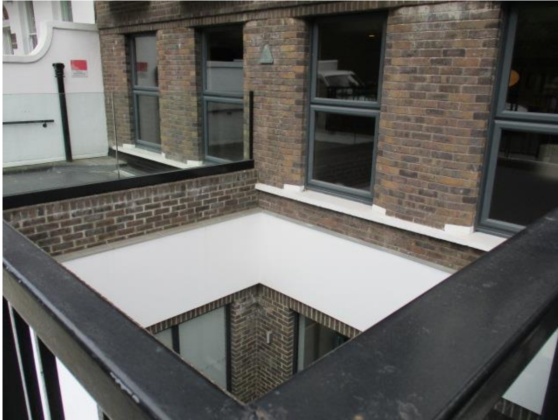
9. Photo showing the lightwell where prefabricated steel ramp will provide level access.
