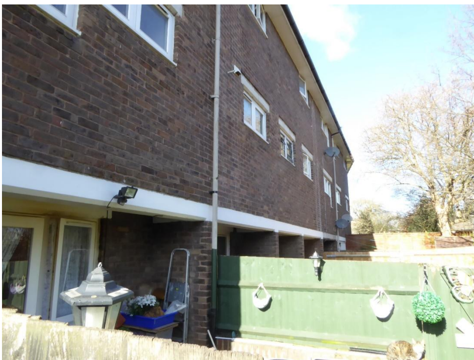
Figure 6. Rear of 81-101 Cressfield Close showing overhang over ground floor windows.
