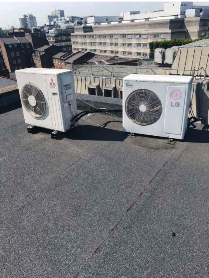
FIGURE 14. EXISTING ROOF-TOP PLANT - VIEWS ACROSS ROOF TO WEST
