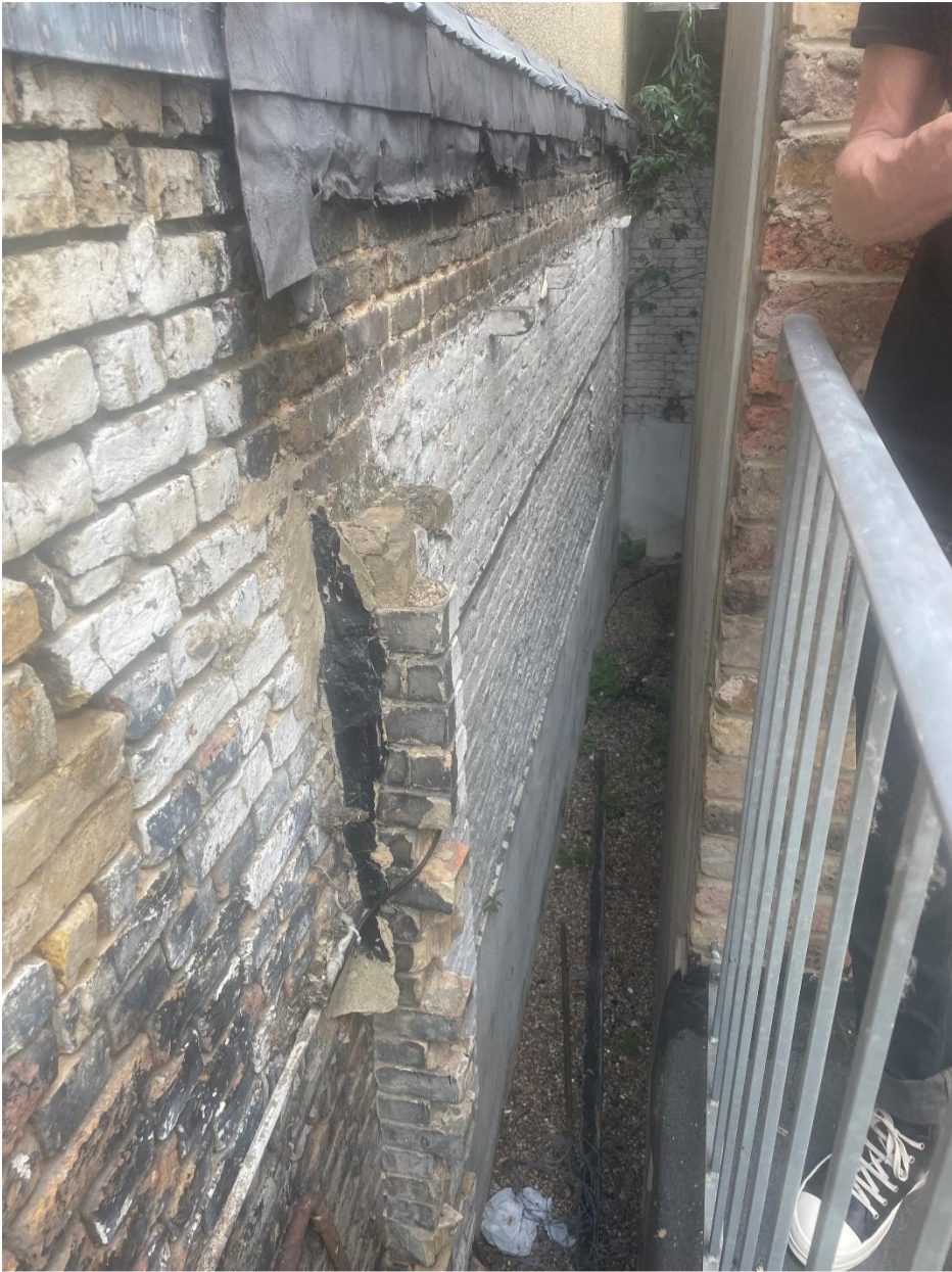
Looking along side gap (north-west) between ground floor unit and boundary wall
