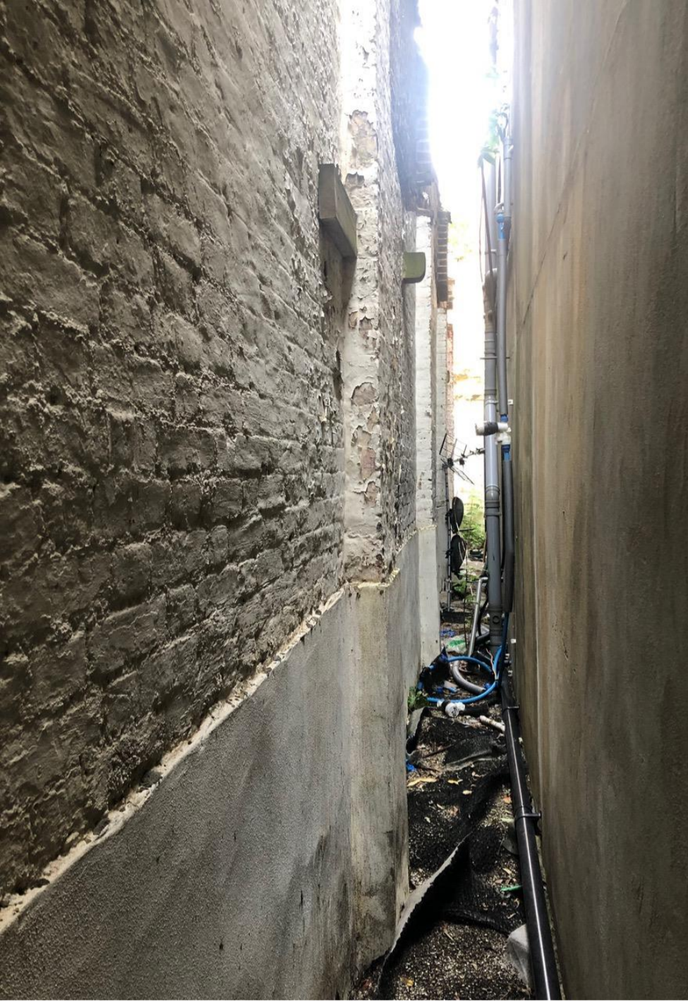
Gap behind rear elevation (North east elevation)
