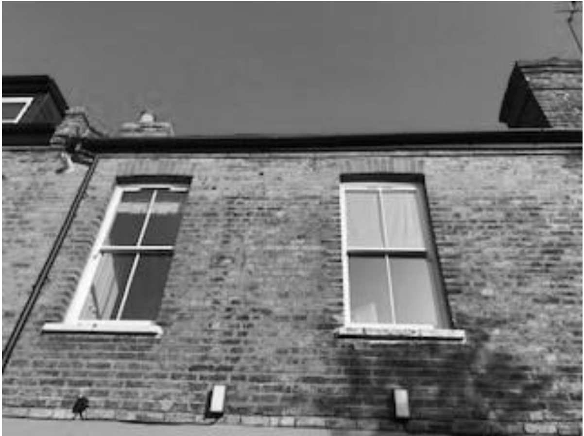
8. View of rear of 26 Constantine Road roof from back of the garden
