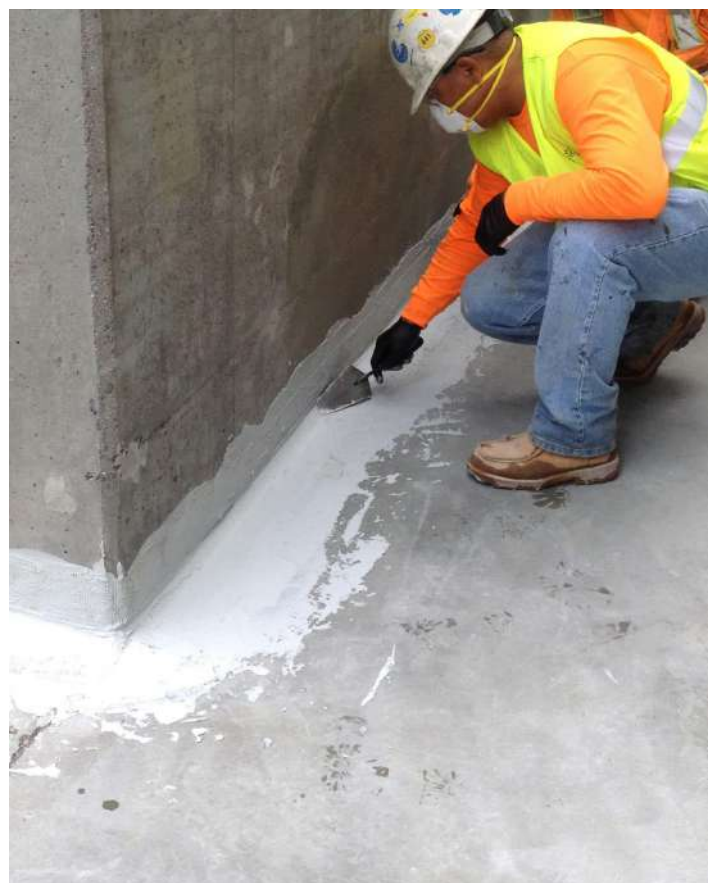
Examples of type A barrier waterproofing applied to wall-floor junction and sprayed on
