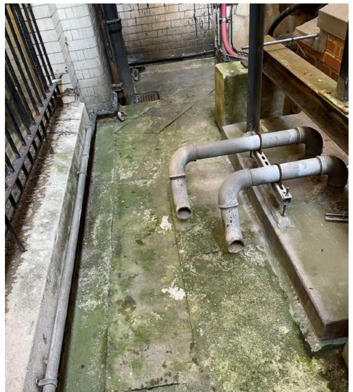
Photo showing area the is regularly flooded resulting in water leakage into the basement. Image shows the misalignment of the drainage gullies and water discharge pipes.
