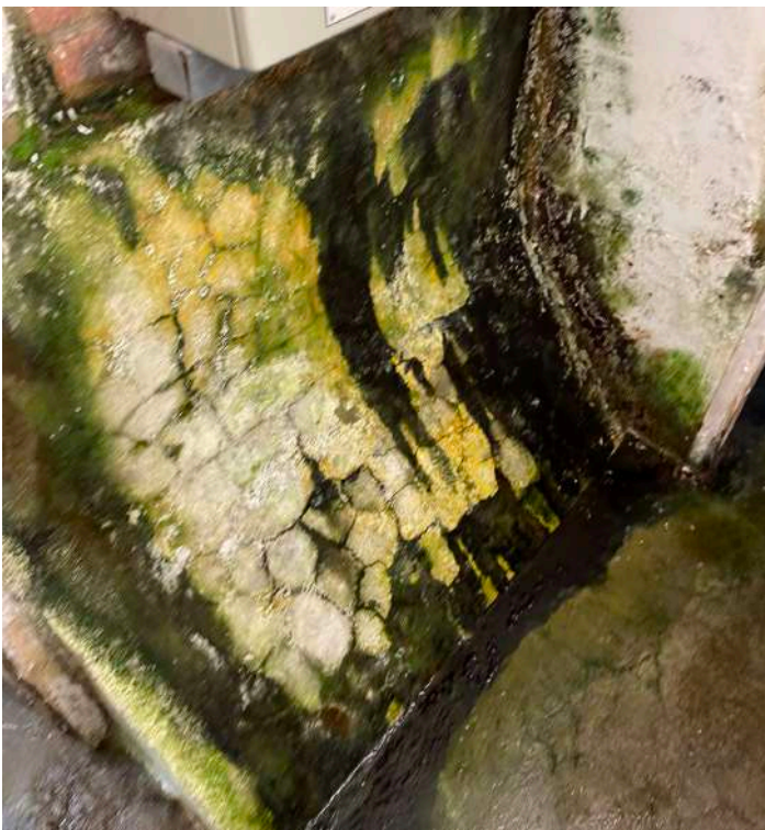
Photo of mould growth on floor and walls
