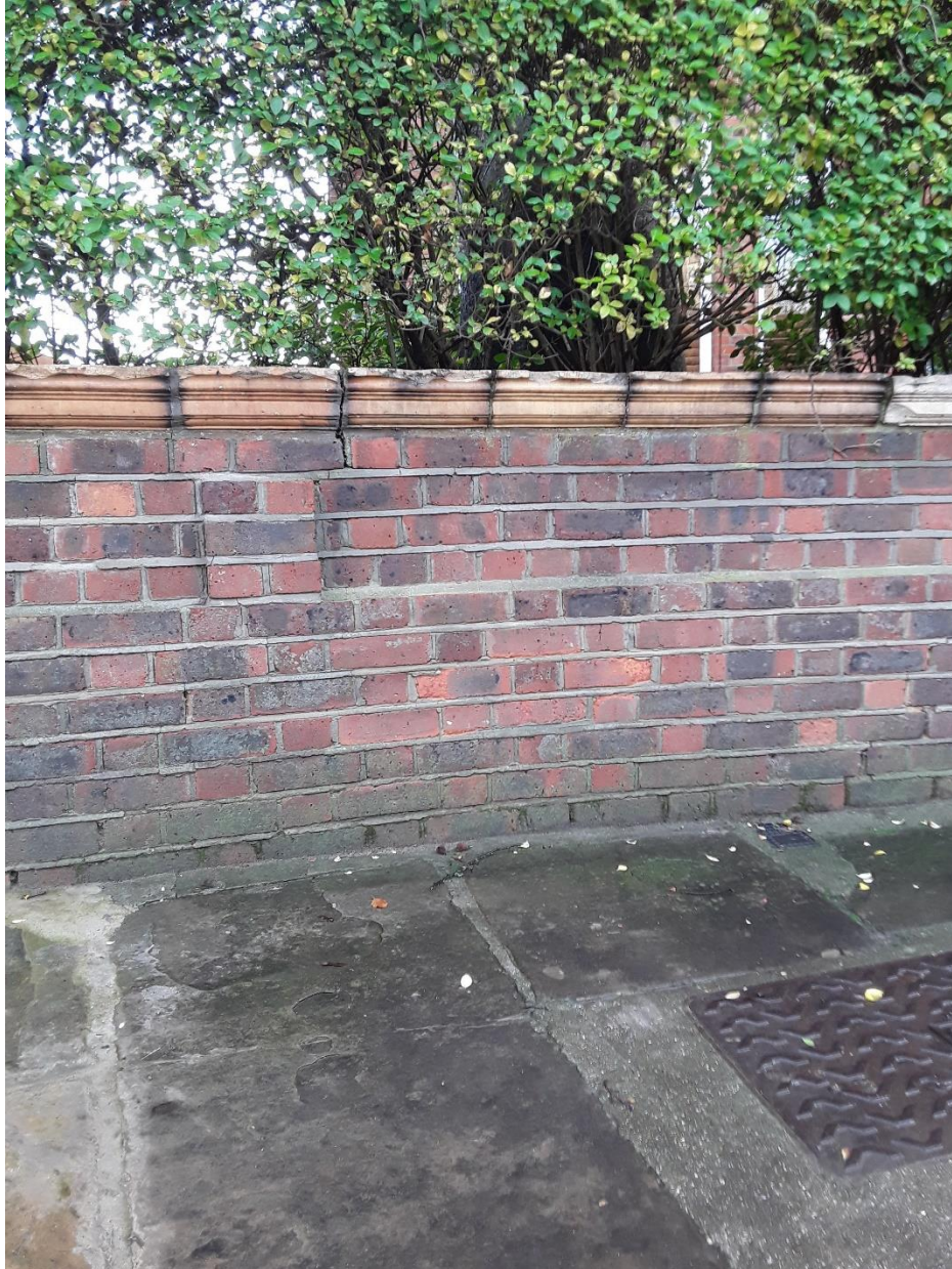
AEL-18129-PIC4 – Showing front boundary wall with crack that will require repair.
