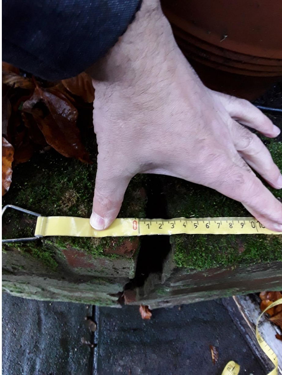
AEL-18129-PIC3 – Showing more significant crack in wall that will require repairing.
