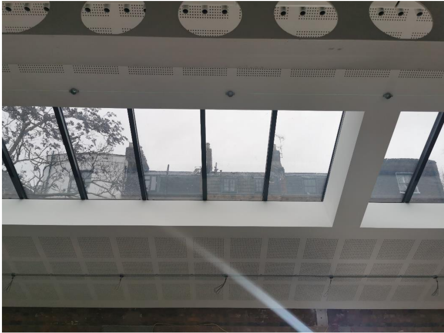
Rooflights on the 2 nd floor of the application site facing Fortess Road
