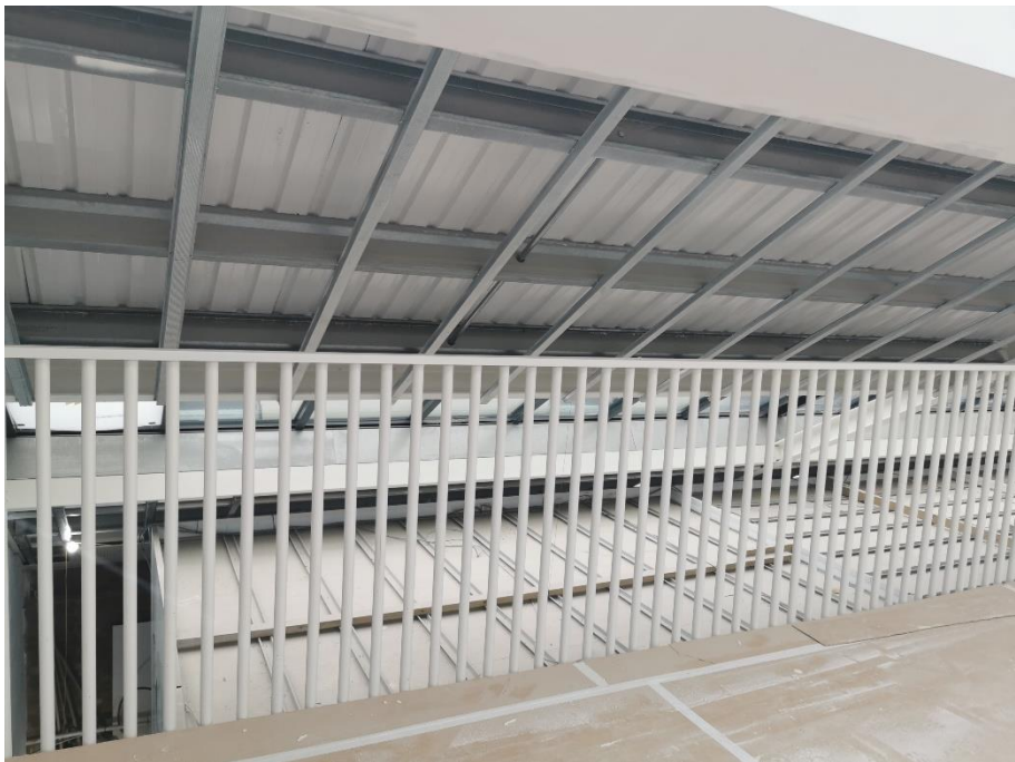
Rooflights on the 2 nd floor of the application, these will remain covered
