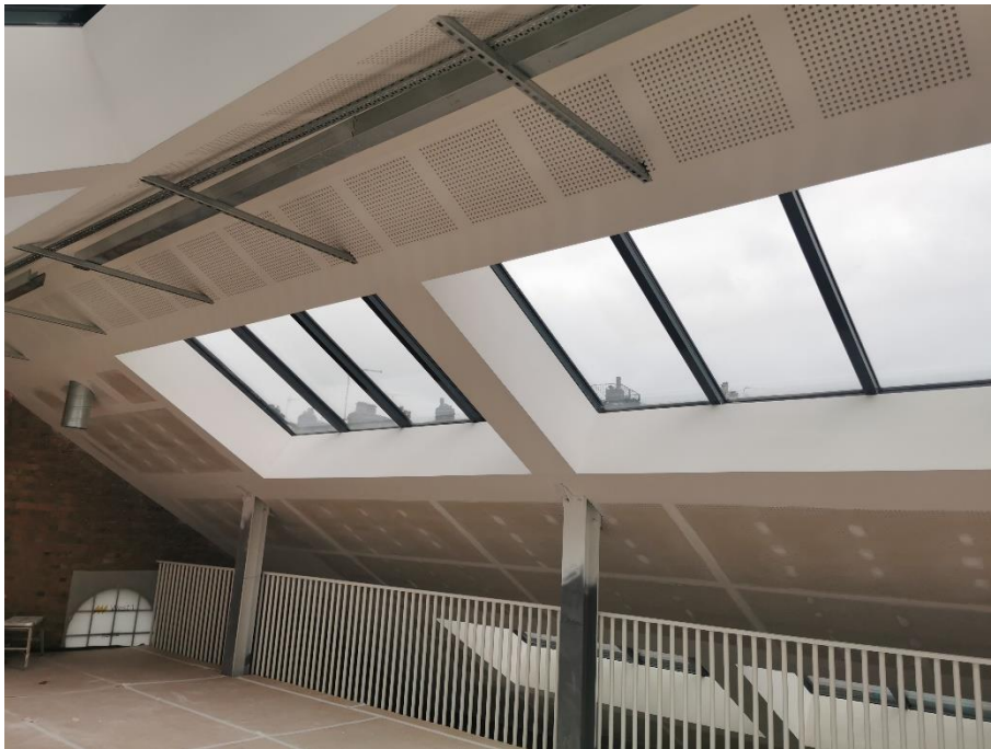
Rooflights on the 2 nd floor of the application site facing Railey Mews
