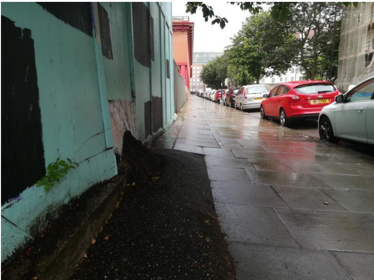
Photo 3: Looking south along the western edge of the Site, showing the area of damaged footpath as caused by T14.
