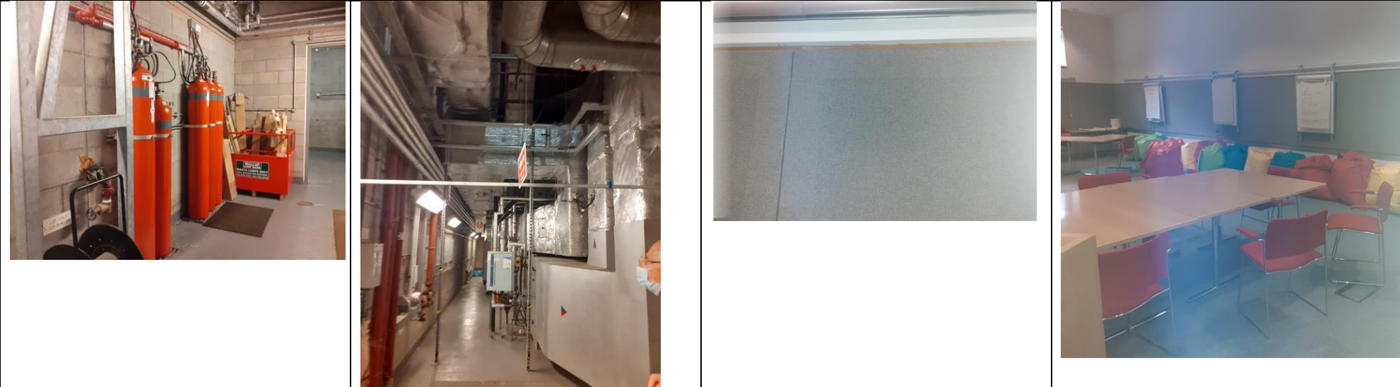
Various plant and equipment, radiators, furniture, Acoustic Boarding
