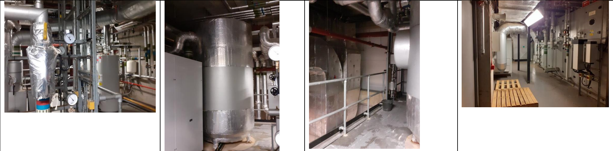
Various plant and equipment, Large calorifier, Invertor AHU,
