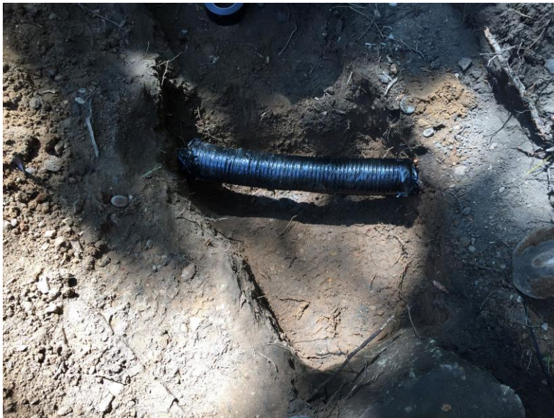
Image 6: Pipe taped over: To prevent cement products from coming into contact with retained roots, the split pipe is taped up (including the ends of the pipe). Root is now ready for further hand excavation or concrete pouring
