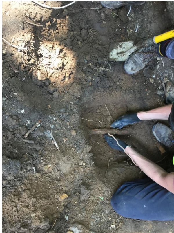
Image 4: hand excavation to retain tree roots: Careful hand excavation or the use of compressed air or vacuum excavation can be used to retain tree roots larger than 25mm diameter
