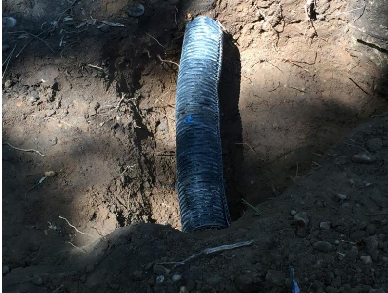
Image 5: flexible split pipe used to protect and retain tree roots: Once exposed by hand digging, tree roots are protected using a flexible split pipe
