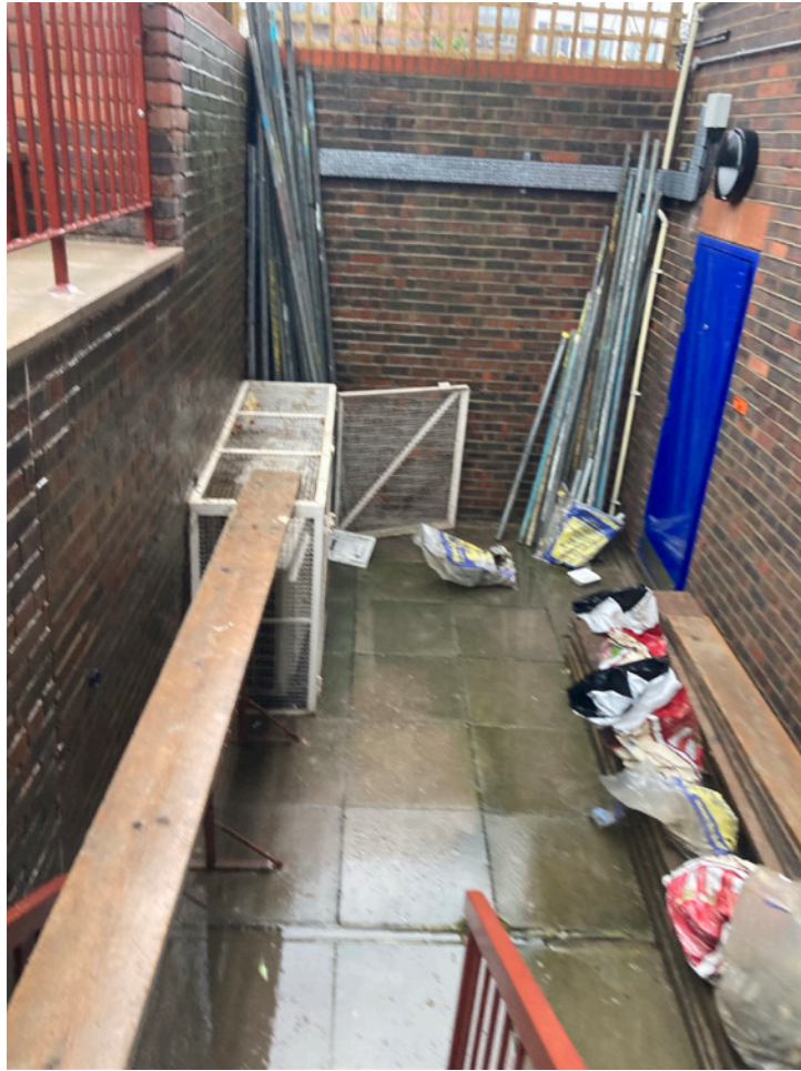
Photo 3: Looking North within lightwell AC unit position shown (metal cage in corner)
