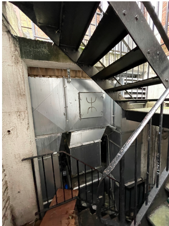
Picture 6: The existing system located under the entrance of flats
