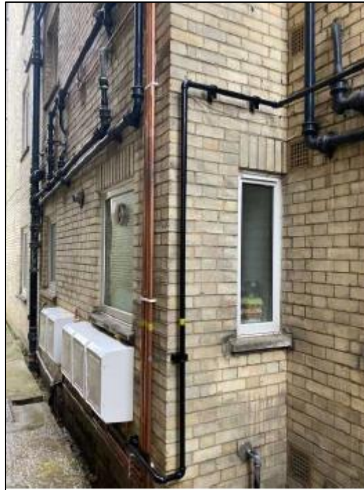
Plate 4: Gas pipework wrapping around the south east facing return elevation of the building
