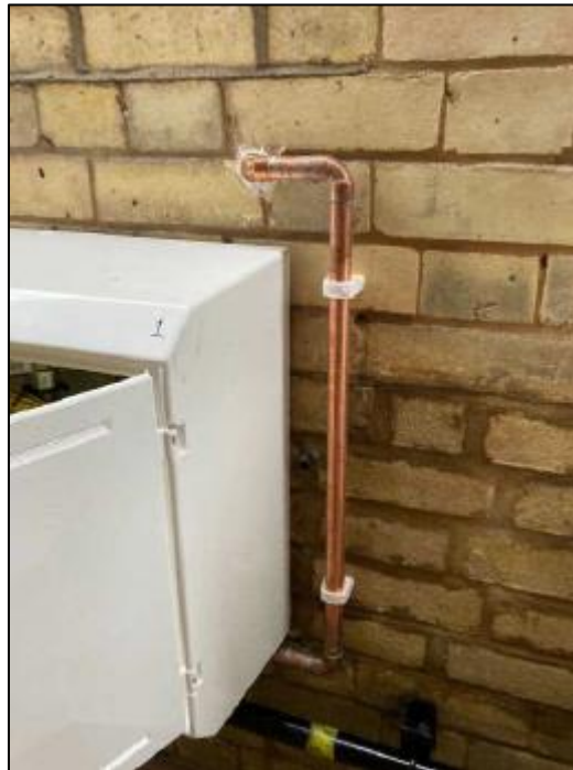
Plate 6: External gas pipework serving ground floor flat at Falmer House flats at 35 Belsize Park
