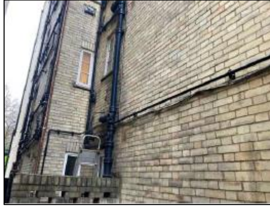
Plate 3: Route of the long section of pipework on the south west facing elevation
