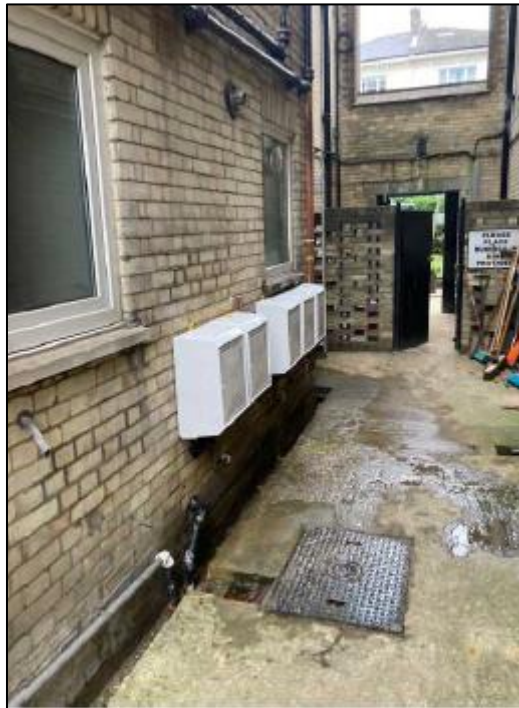
Plate 5: Route of horizontal pipework including meter boxes on the south west facing elevation.
