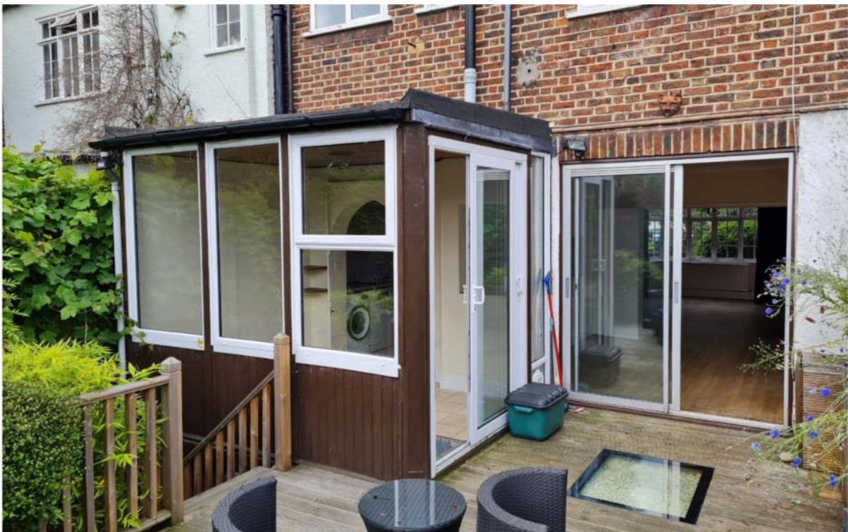
4. Photo of rear elevation showing existing half width rear extension (on boundary with no. 21)
