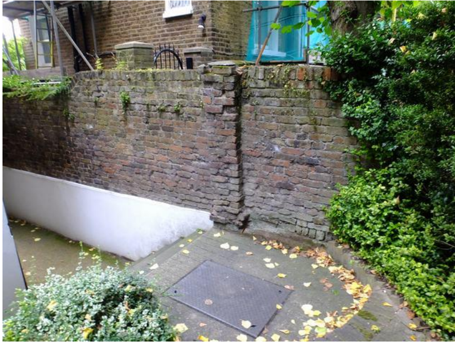
Image 11 Inspection cover for existing services, so roots likely to have been restricted or severed.
