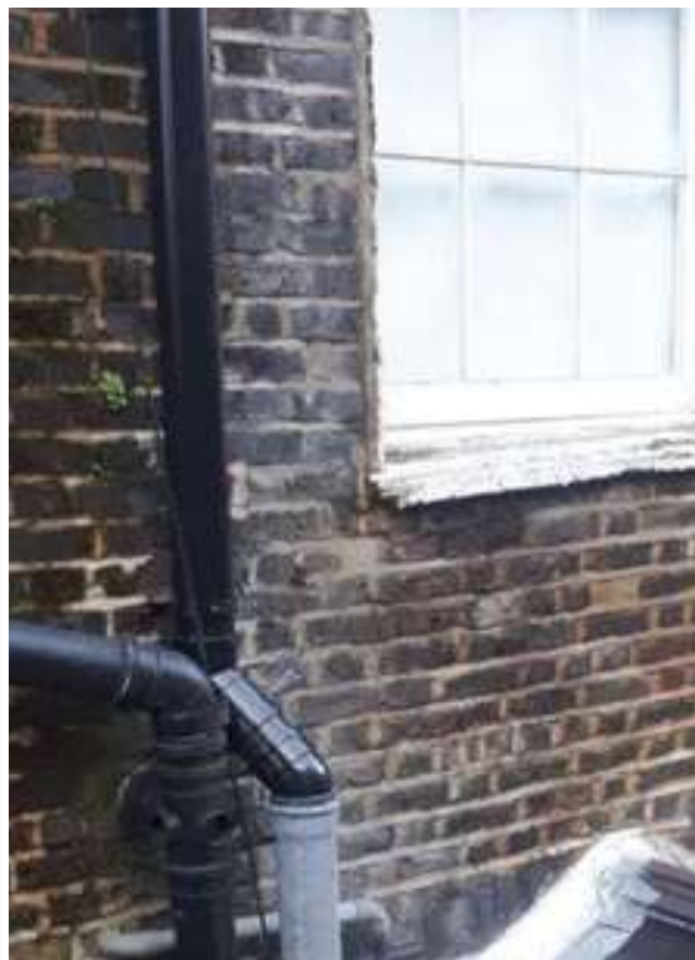
5.02 First floor flat's rear window with damaged sill
