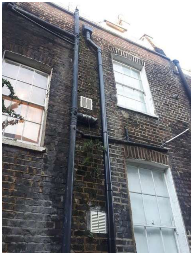
5.01 Back elevation in need of maintenance
