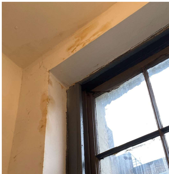
5.04 Water ingress around the staircase's window
