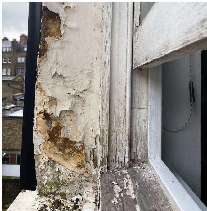
5.03 Condition of first floor flat's rear window
