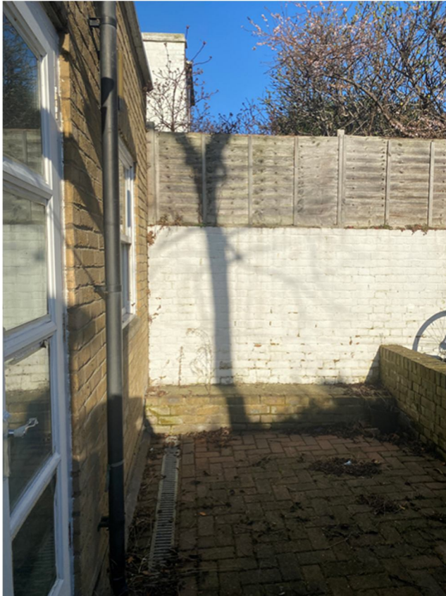
Photo: Boundary wall with fence shown of 70A & 72 Marquis Road exceeds 9ft in height, shown in photo and highlighted in yellow above (drawing)
