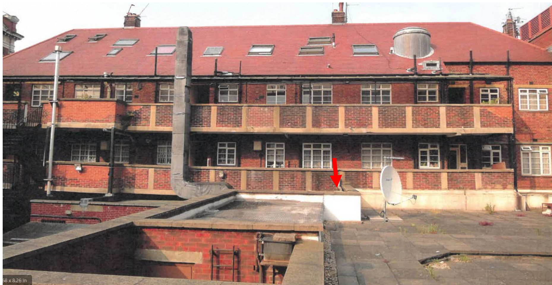
205-207 Haverstock Hill – Location Details of Air Con Units
