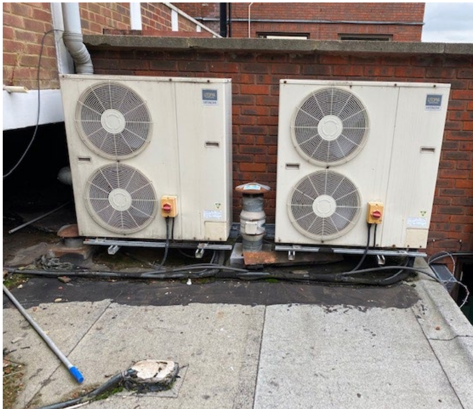
205-207 Haverstock Hill – Location Details of Air Con Units
