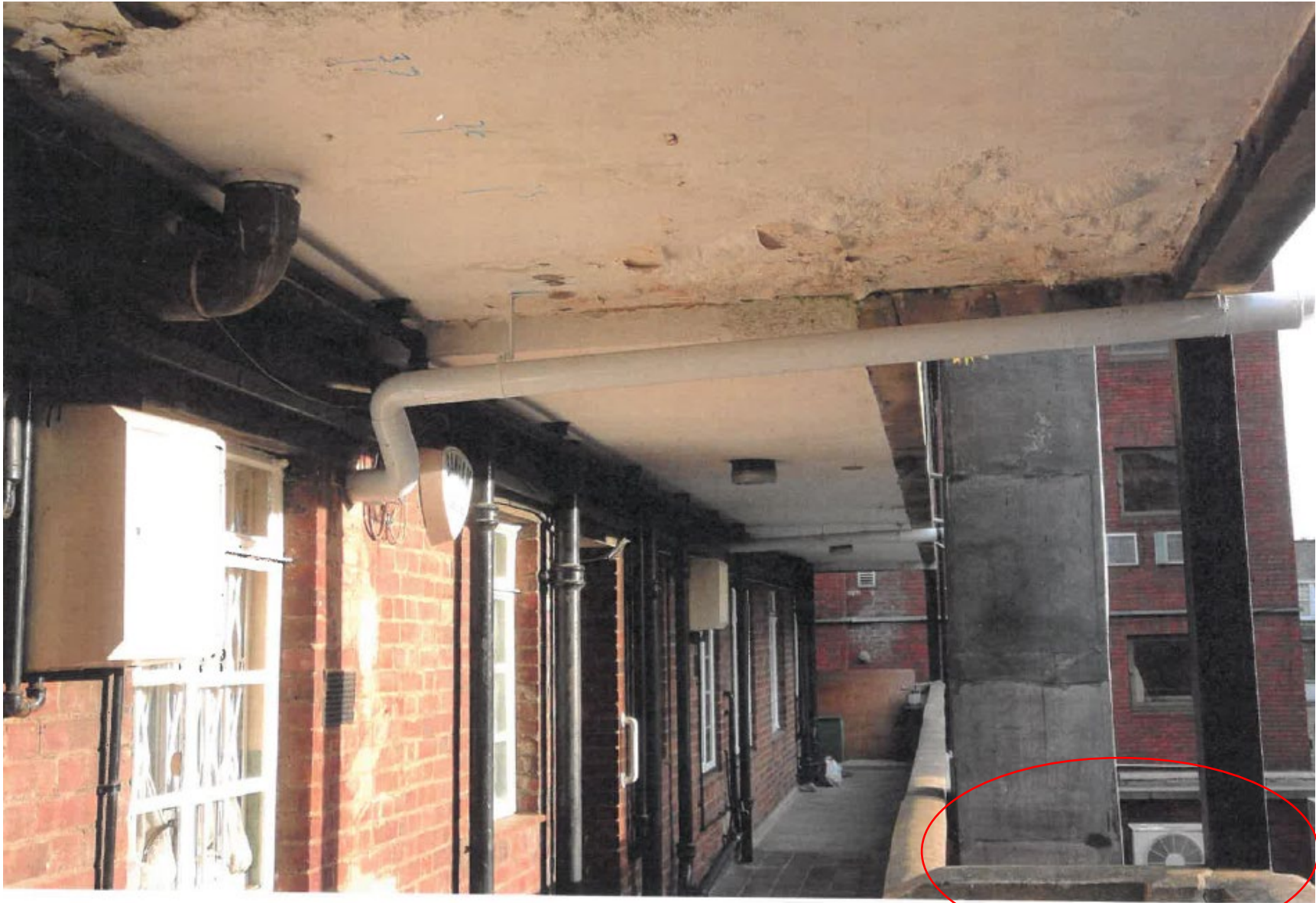
205-207 Haverstock Hill – Location Details of Air Con Units
