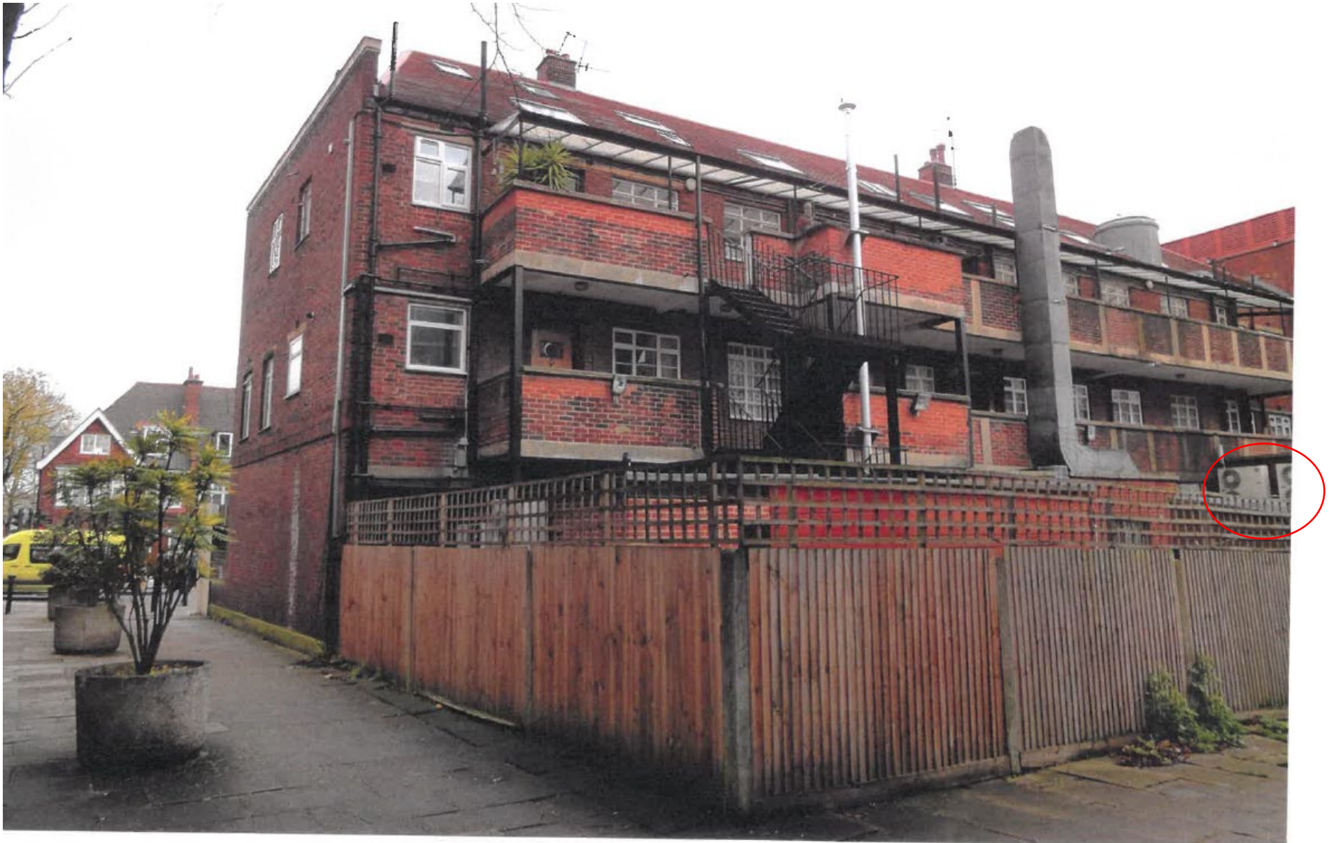
205-207 Haverstock Hill – Location Details of Air Con Units
