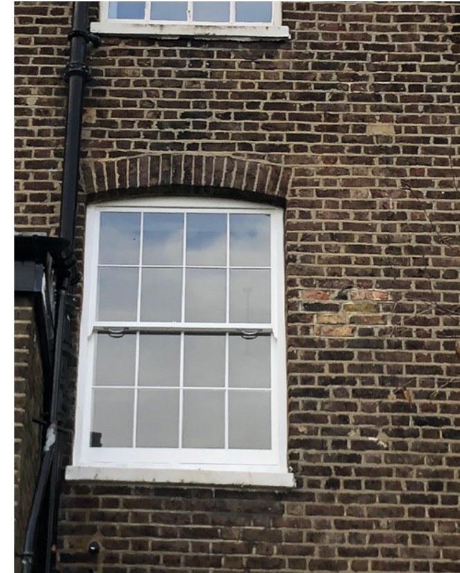
Images of rear exterior and existing pointing conditions - poor, weathered and dirty.
