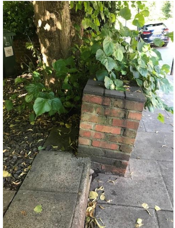
Photograph 2: Showing deflection of front wall, possibly as a result of trees T4 and T5.
