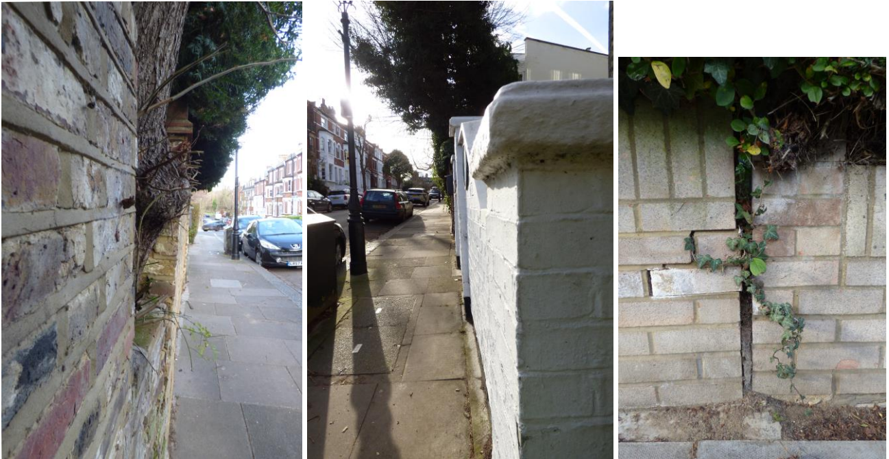
4: View down Pilgrims Ln from above T1 5: View up Pilgrims Ln from below T2 6: Movement joint in wall near corner
