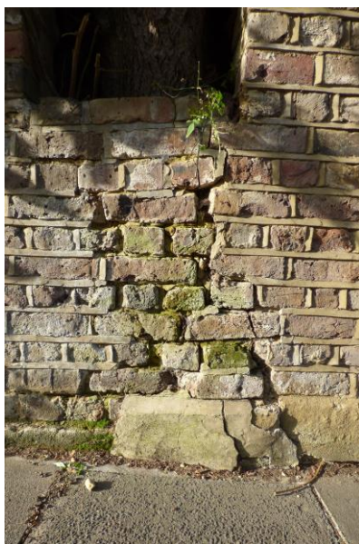
2: Wall & cement pointing failure
