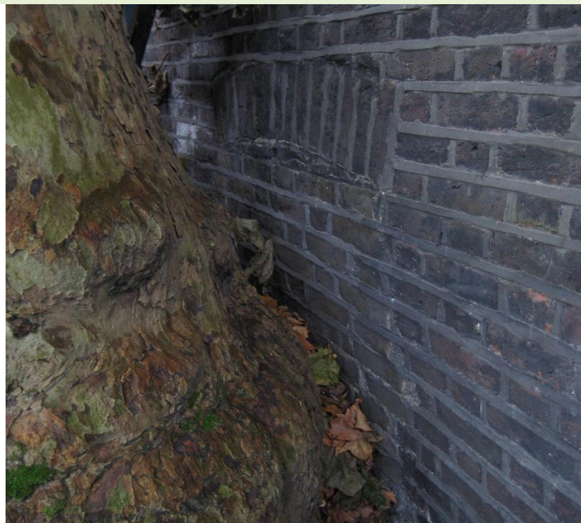
Image 2 – T1 showing direct contact with the rear of the property. Only removal of T1 & T2 will remove this issue
