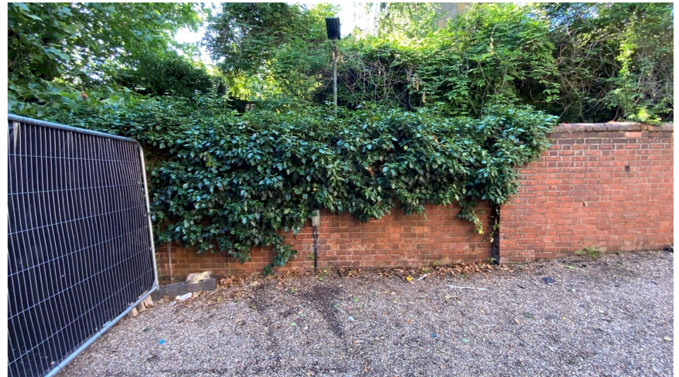
Figure 34: North elevation of the boundary wall taken from the driveway of 82 Fitzjohn's Avenue showing the wall covered in significant quantities of foliage. A defunct light and cabling dating from the middle of 20 th century is visible.
