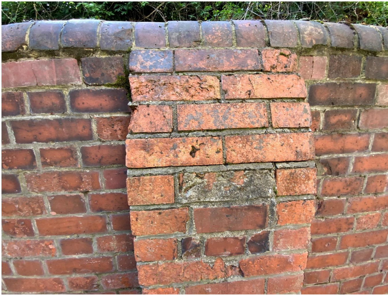
Figure 30: Photograph of the additional buttress showing poor quality cement mortar that is beginning to fail, cement mortar has been poorly applied to the brickwork in the main wall also and there are signs of decay.
