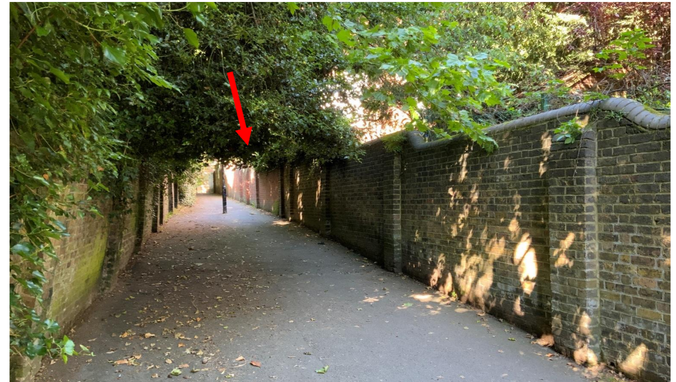
Figure 40: Photo looking westwards down Spring Walk towards Fitzjohn's Avenue. The red brick section of wall that is proposed to be dis-assembled and re-assembled is on the far right annotated with a red arrow.
