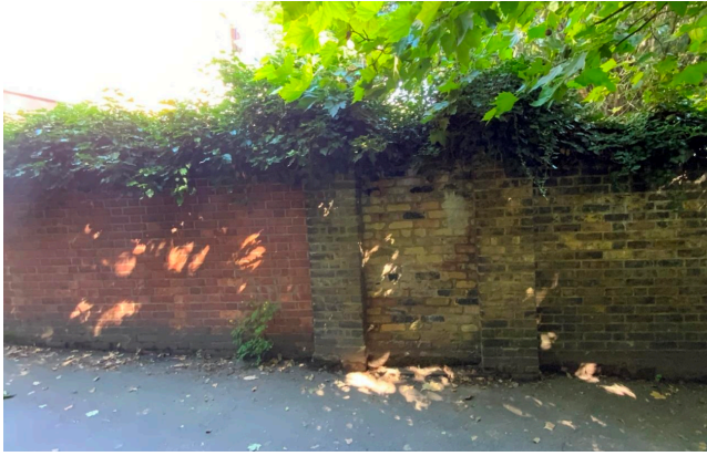
Image 04 - View of the wall from Spring Walk indicating where the original wall meets the new section of the wall to be disassembled
