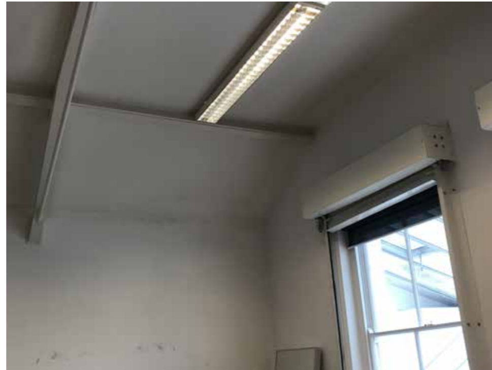
Low quality surface mounted lights
