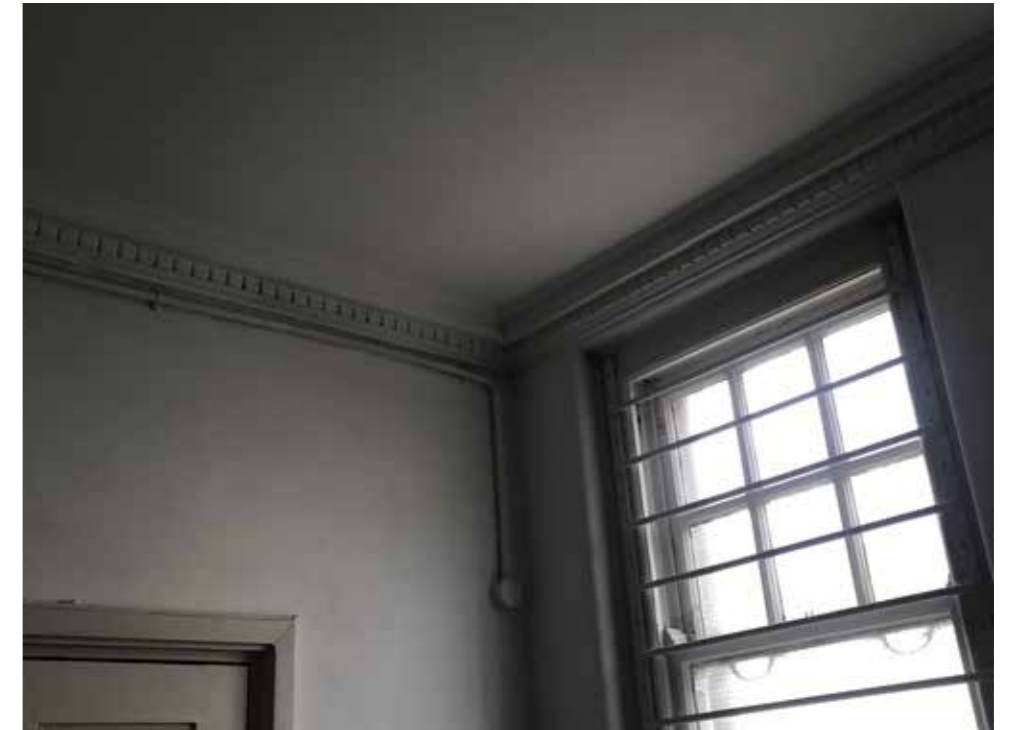
Existing exposed services adjacent to historic features
