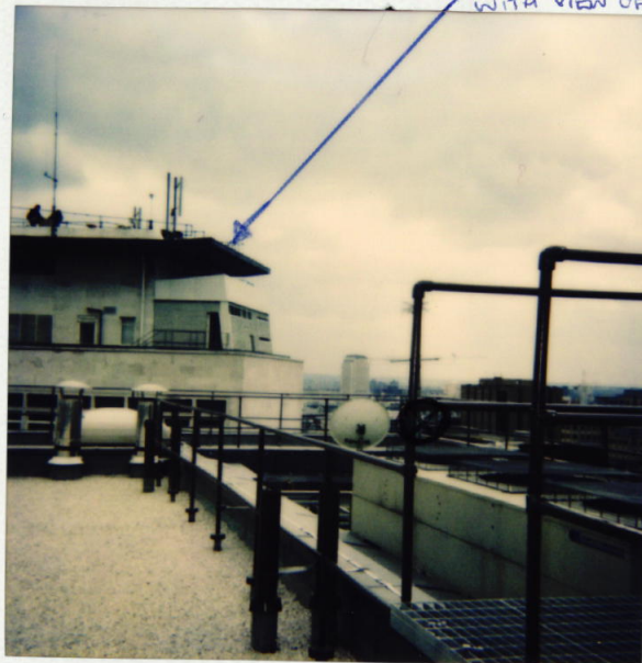
15-19 BLOOMSBURY WAY view towards back of dish location -showing top of depressed roof plant machinery
