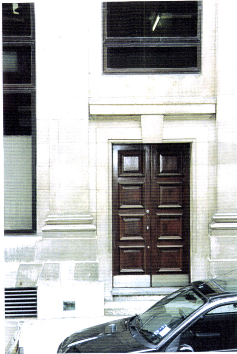
EAST ELEVATION (Service Door to be removed and replaced with window to match)
