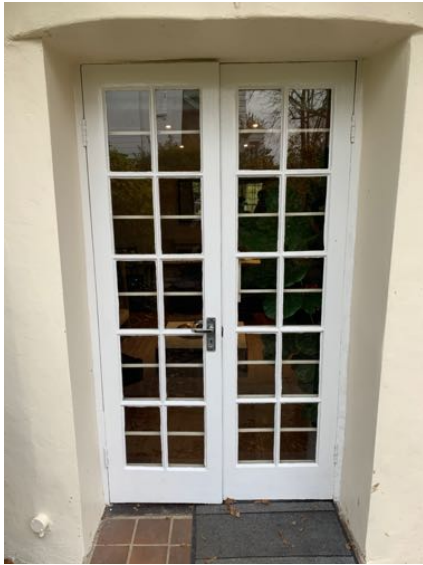
Rear elevation (2) non-original double doors to be replaced
