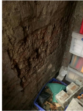
Images showing brick erosion
