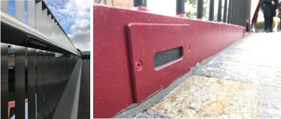
Photograph 3 and 4: Lighting on Somers Town Bridge and on Kings Cross Bridge 2
