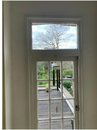
Second floor terrace to be retained and railings added for building regulations
