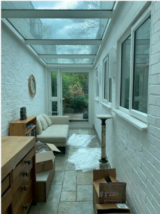
Ground Floor side extension to be replaced
