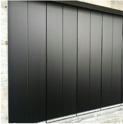
Figure 1 Consented scheme (ref: 2020/1945/P) with polyester powder coated, aluminium-clad front door and gate; seams at wider intervals (approx. 900mm).
