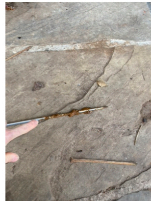
Probe showing limited extent of open decay (entering 120-140mm maximum)
