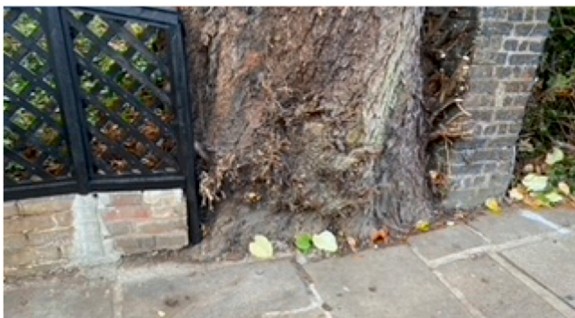
Base of tree within edge of highway as viewed in a north westerly direction
