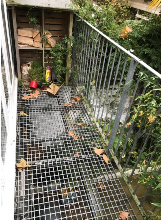
Plate 3: Ground floor rear steel balcony (to be removed)
